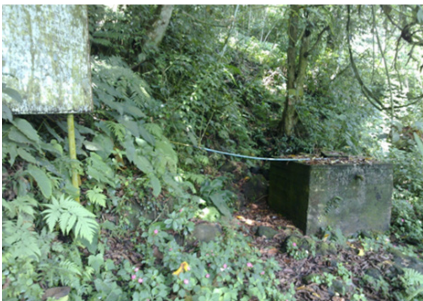
Figure 3.3. Spring water storage tank in Barangay Bukal, Nagcarlan
