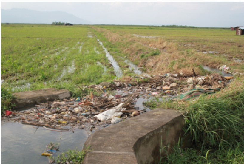
Figure 3.4. Garbage-filled irrigation canal in Brgy. San Pablo Sur, Sta. Cruz
